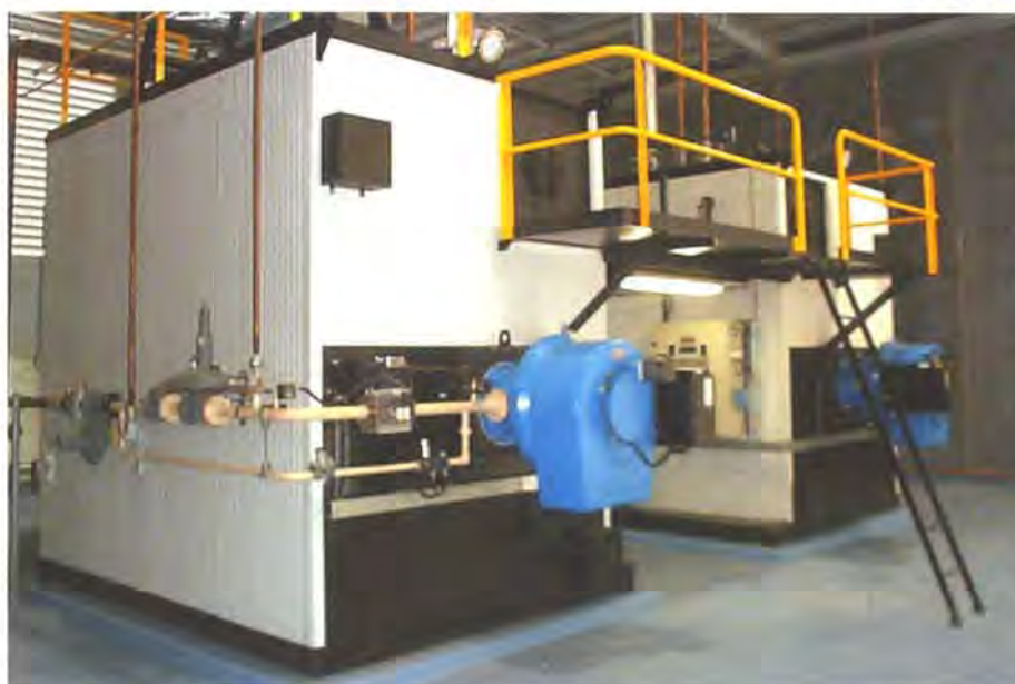
Two 350WT Watertube Steam Boilers
